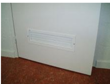
Doorstroomopening in deur
